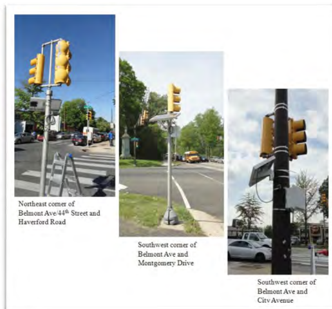
Figure 1 – Typical Solar Powered BlueTOAD™ Device Installation
